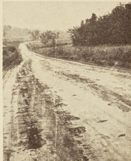
SURFACE PITTED AND RAVELED
